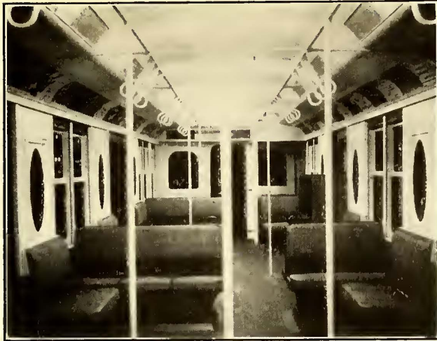
NEW YORK MUNICIPAL CAR—FIG. 15—LIGHTING EFFECT OF INSTALLATION SHOWN IN FIGS. 1 AND 9
