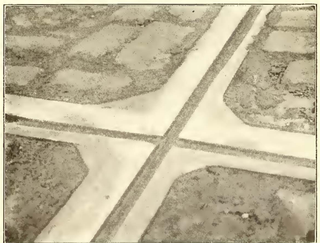
MANGANESE STEEL CROSSINGS—FIG. 5—BEGINNING OF DEPRESSION, WENTWORTH AVENUE AND FIFTY-NINTH STREET, CHICAGO
