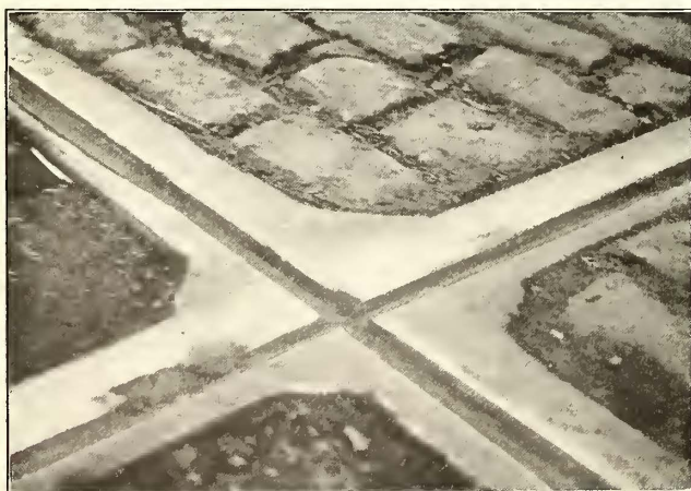
MANGANESE STEEL CROSSINGS—FIG. 7—PIECE SPALLED OUT OF DEPRESSION, WENTWORTH AVENUE AND FIFTY-NINTH STREET, CHICAGO
