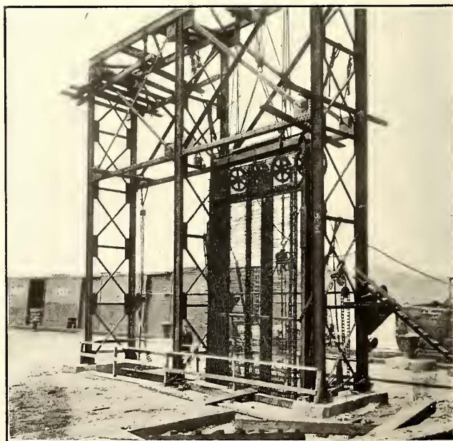
INTERBOROUGH POWER PLANT—FIG. 12—REVOLVING INTAKE SCREEN
