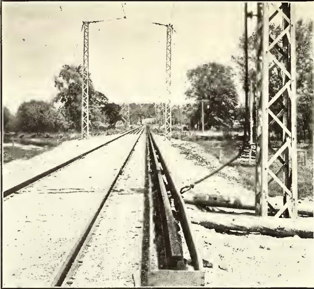
MICHIGAN 2400-VOLT LINE—VIEW SHOWING CHANGE FROM THIRD RAIL TO OVERHEAD CONTACT WIRE
