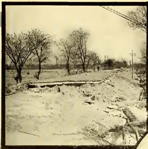
Showing destruction of Levee Road caused by flood.
