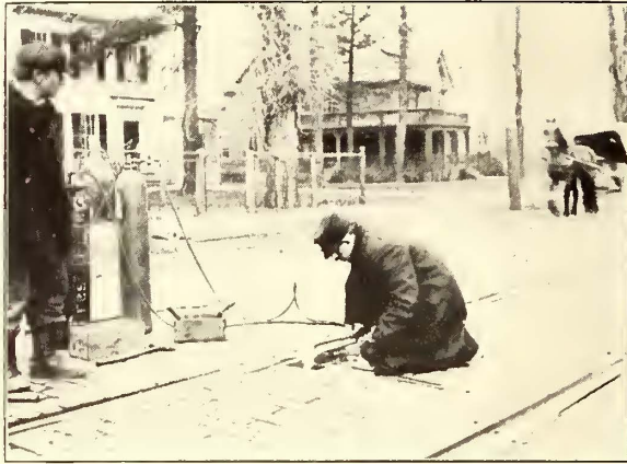
Building up a guard rail with the Prest-O-Lite welding outfit. This simple operation obviates expensive disorganization of traffic and loss of time that replacing by any other method would require.
