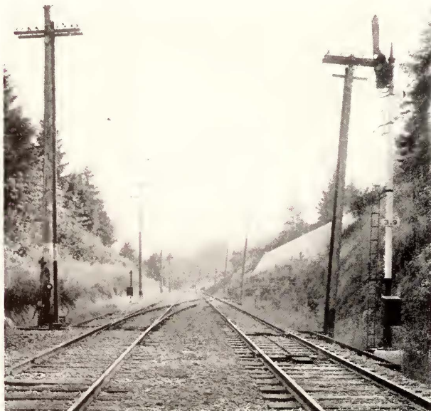
Top-Post Mechanism of A.C. Track Circuit Signals at Cross-over on Double-Track Section, Oregon Electric Railway
