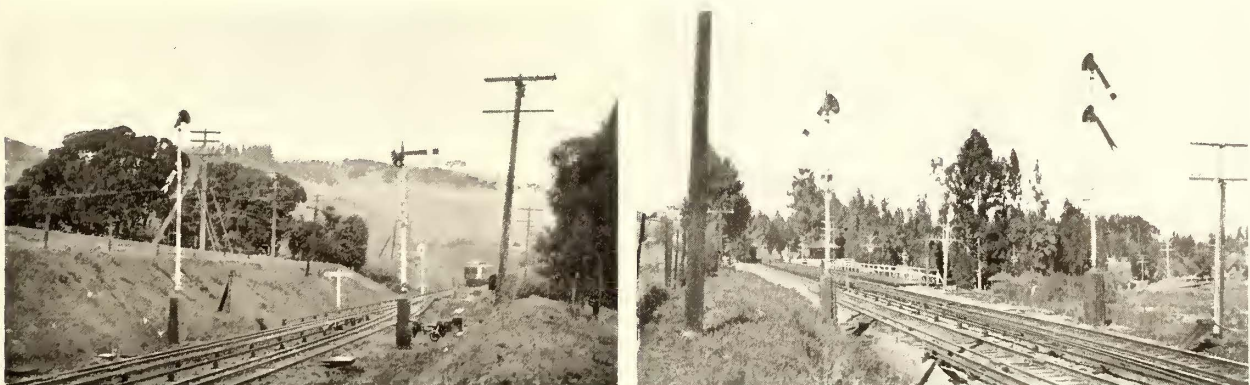
Twelve-Year-Old A.C. Track Circuit Signals at East Portal of Corte Madera Tunnel
