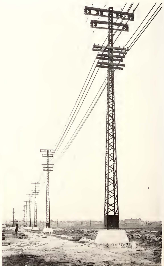
Transmission Line, Oakland Electrification
