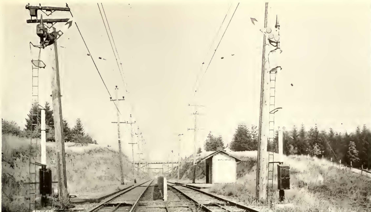
Top-Post Mechanism of A.C. Track Circuit Signals on Double-Track Section at Maplewood, Oregon Electric Railway
