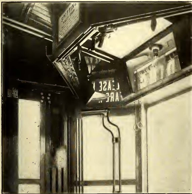
BAY STATE CAR—SIGN BOXES AND SWITCHES ON HEADER OVER MOTORMAN'S COMPARTMENT
