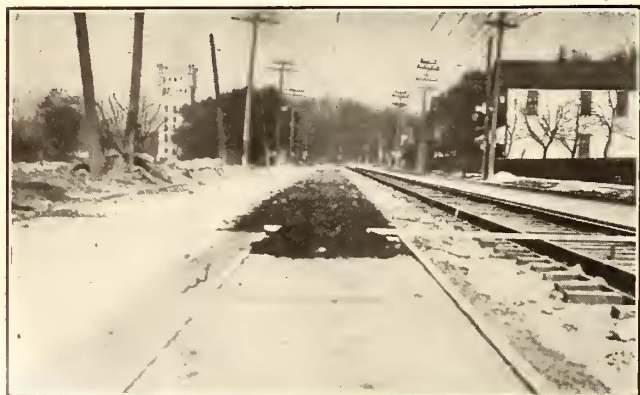
CONCRETE PAVEMENT—MOIST EARTH COVERING TO PRE- VENT TOO RAPID DRYING OF CONCRETE
