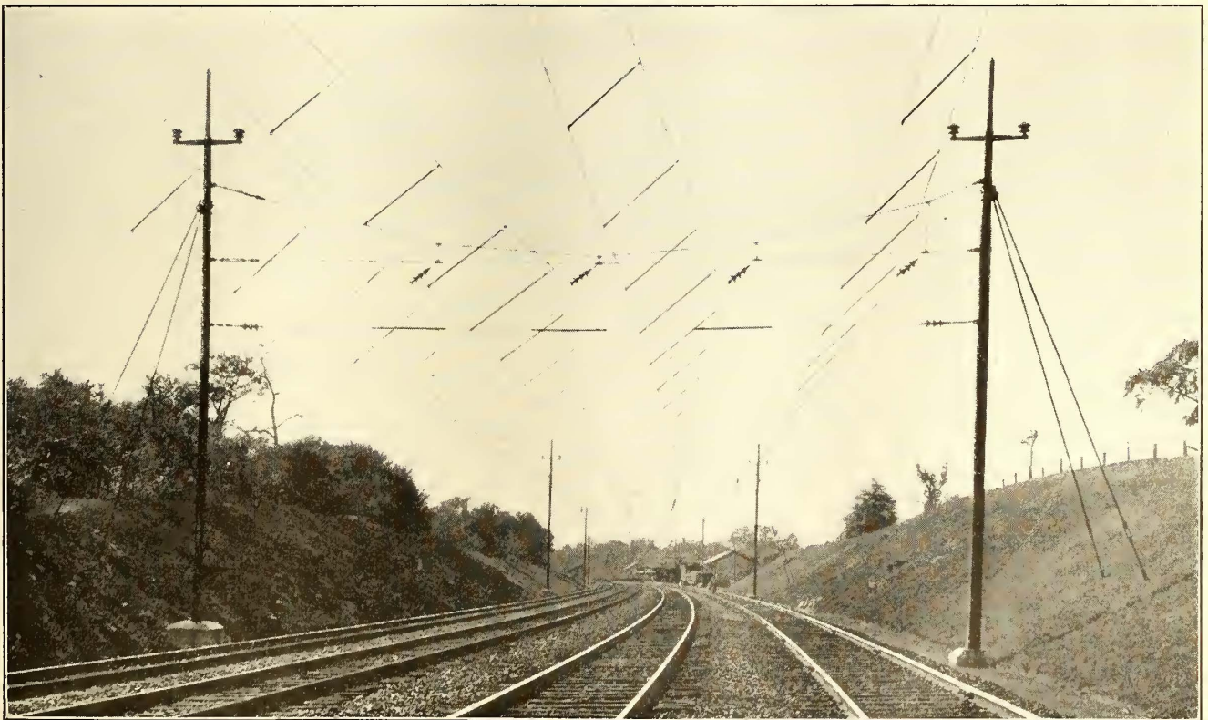
PHILADELPHIA-PAOLI ELECTRIFICATION—TYPICAL CATENARY CONSTRUCTION ON SHARP CURVE
