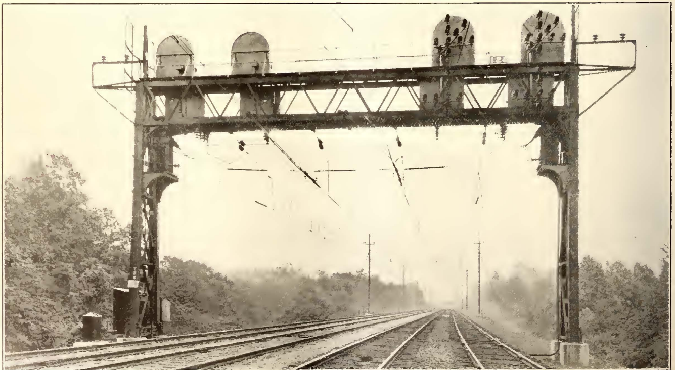
PHILADELPHIA-PAOLI ELECTRIFICATION—TYPICAL ANCHOR AND SIGNAL BRIDGE LOCATED AT END OF CURVE; TRACK-BOOSTER TRANSFORMERS MOUNTED AT BOTH SIDES
