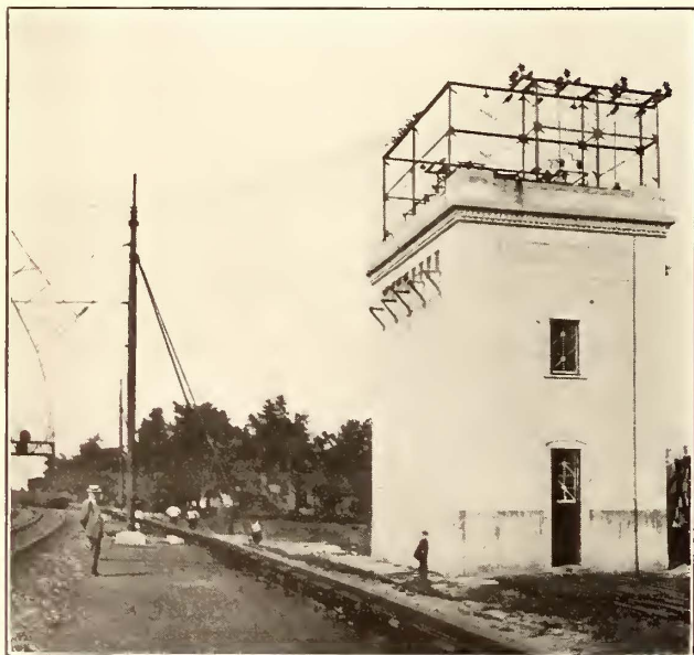
PHILADELPHIA-PAOLI ELECTRIFICATION—VIEW OF SUBSTATION SHOWING ARRANGEMENT OF 44,000-VOLT TRANSMISSION CABLES AND 11,000-VOLT FEEDERS
