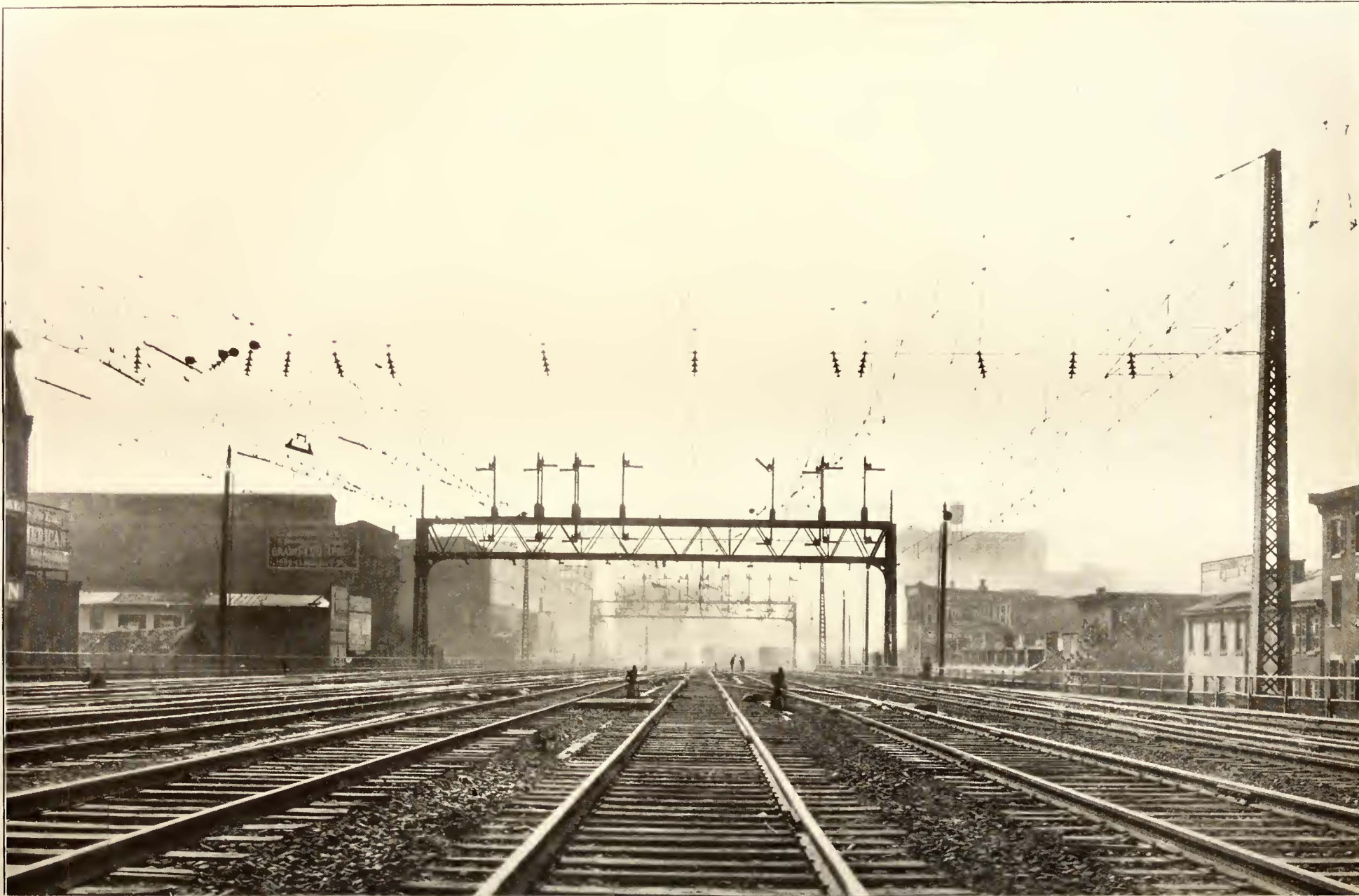
PHILADELPHIA-PAOLI ELECTRIFICATION—VIEW OF CROSS-CATENARY OVER NINE TRACKS, SHOWING READY VISIBILITY OF SEMAPHORE SIGNALS NOTWITHSTANDING COMPLICATED OVERHEAD CROSS-OVERS
