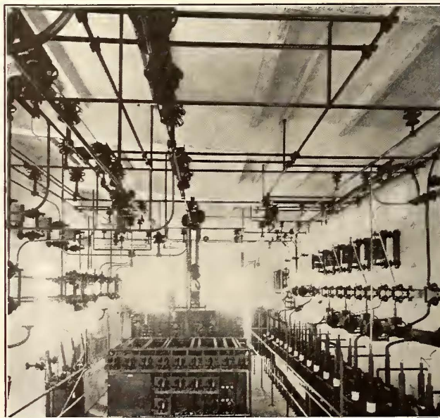
PHILADELPHIA-PAOLI ELECTRIFICATION—INTERIOR VIEW OF SECOND FLOOR OF TYPICAL SUBSTATION SHOWING BUSBAR AND SWITCHING EQUIPMENT
