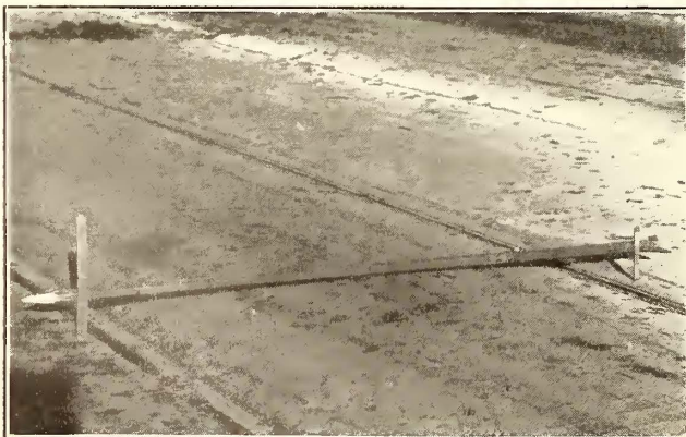
FROST-HEAVED WOOD-BLOCK PAVING
