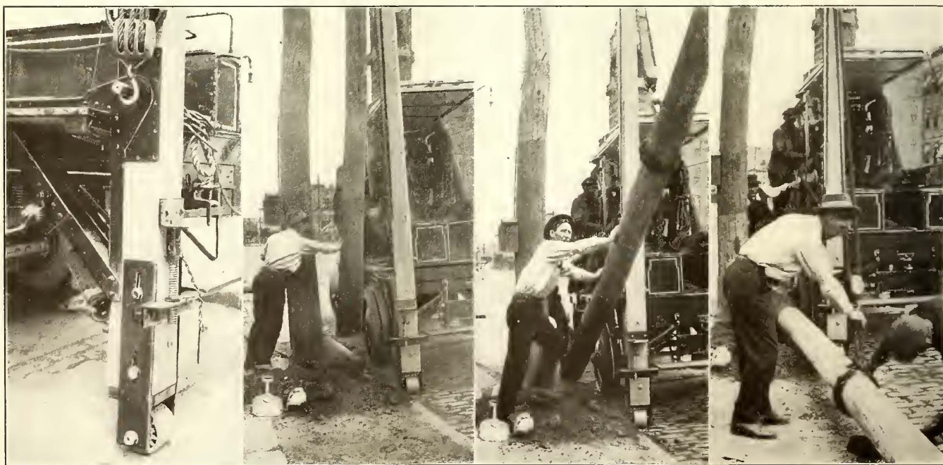
THIRD AVENUE LINE TRUCKS—WOOD POLE REMOVAL: TRUCK IN POSITION READY FOR HOISTING, POLE HOISTED AND CLEAR OF GROUND, LOWERING AWAY AND JOB COMPLETE, ALL AT THE RATE OF FIFTEEN TO TWENTY PER HOUR
