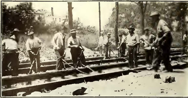
Pneumatic Tie Tamping—Fig. 3—Six Machines in Use on Double Track Extension in East Orange, N. J.
