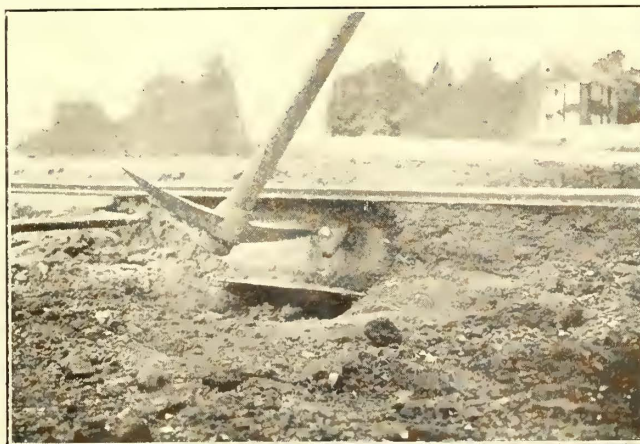
VIEW OF CLAY PICK DRIVEN THROUGH CORRODED RAIL WEB
