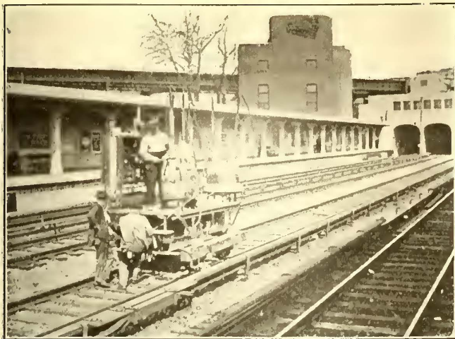
THIRD-RAIL BONDING—ELECTRIC FURNACES FOR HEATING COPPER ERECTED ON SPECIAL TRUCK HAVING THIRD-RAIL SHOE
