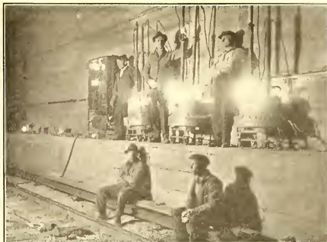
THIRD-RAIL BONDING—ELECTRIC FURNACES FOR HEATING COPPER BEING OPERATED IN SUBWAY WHERE CLEARANCE IS SMALL
