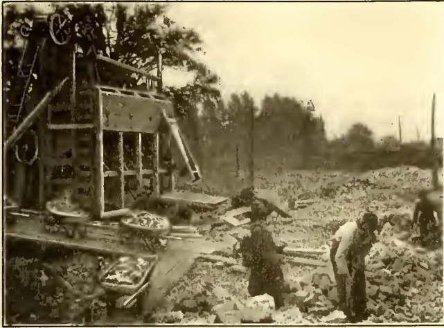
STORAGE YARDS—FIG. 20—STONE CRUSHER IN USE IN YARD OF NEW YORK STATE RAILWAYS, ROCHESTER, N. Y.
