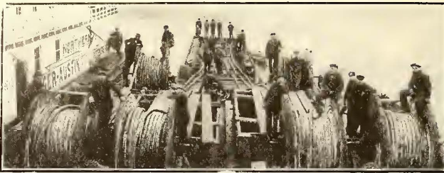
Duquesne Light Co. Laying 11,000-volt Sub-Marine Cables, made by Standard Underground Cable Co., Across Ohio River at Pittsburgh.
