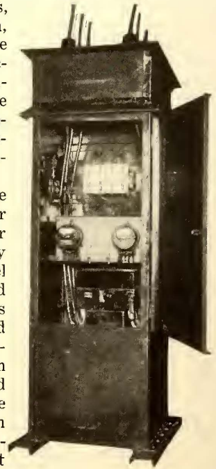
INSIDE VIEW OF PORTABLE SWITCH-HOUSE
