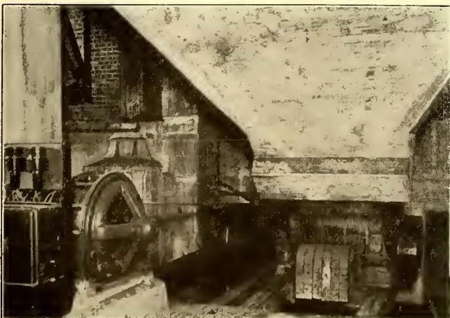
COAL AND ASHES HANDLING—COAL CRUSHER AND MOTOR, TONAWANDA PLANT
