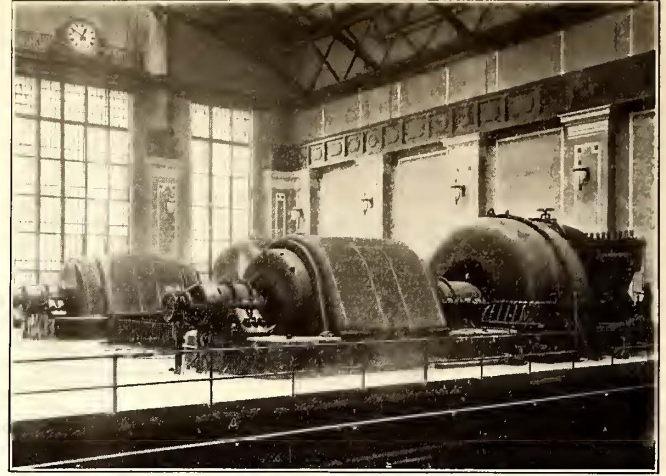
NEW PUBLIC SERVICE POWER PLANT—25,000-KVA. TURBO-GENERATORS, PRESENT EQUIPMENT OF TURBINE ROOM
