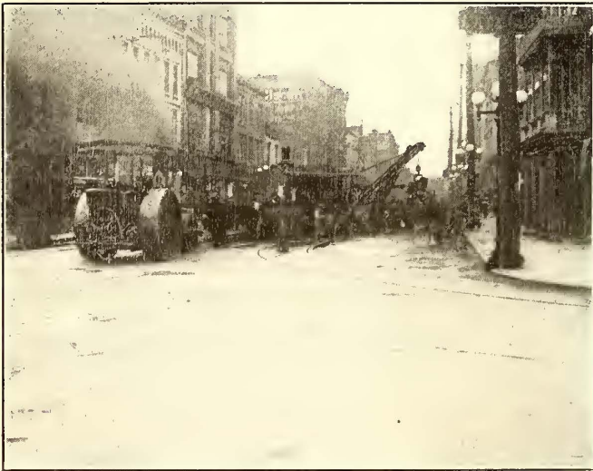
ELMIRA TRACK RECONSTRUCTION—FIG. 8—STEAM SHOVEL AND STEAM ROLLER AT WORK; STRETCH OF FINISHED TRACK IN FOREGROUND
