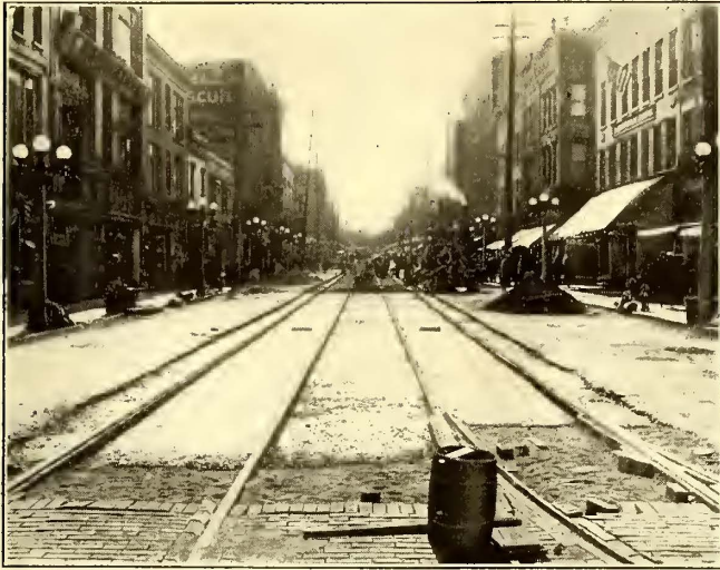
ELMIRA TRACK RECONSTRUCTION—FIG. 11—CONCRETE FOUNDATION, SAND CUSHION AND SPECIAL FILLER PAVING BLOCKS NEXT TO RAILS ON INSIDE OF TRACK
