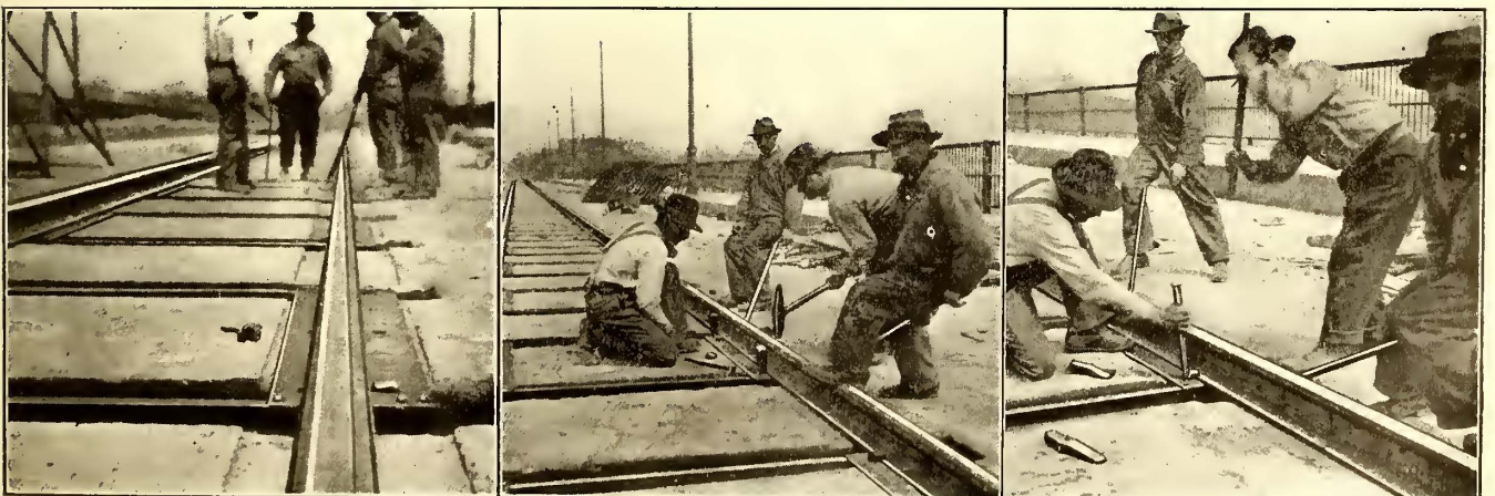
CLEVELAND BRIDGE TRACK CONSTRUCTION—RAIL ON TIE BEFORE APPLICATION OF FASTENING; FORCING RAIL UNDER ONE SET OF CLIPS; FORCING SECOND CLIP AGAINST RAIL BASE BEFORE DRIVING WEDGE
