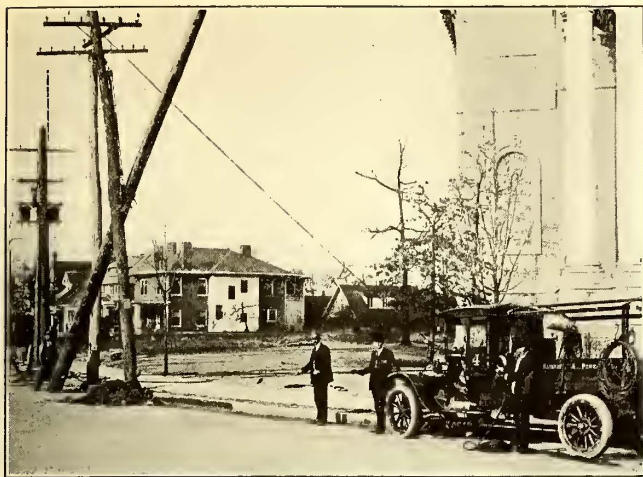
ONE OF THE 2-TON MOTOR TRUCKS USED FOR HANDLING AND SETTING POLES
