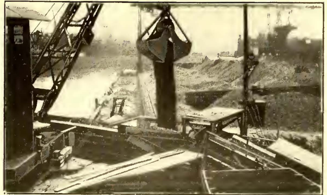
MILWAUKEE COAL HANDLING—BELT CONVEYOR AND LOCOMOTIVE CRANE DUMPING COAL INTO CRUSHER HOPPER SIMULTANEOUSLY
