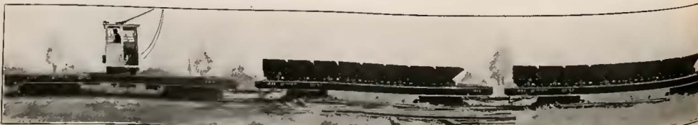
DENVER TRAMWAY CONCRETING TRAIN. ONE FLAT CAR REMAINS WITH THE MIXER WHILE
