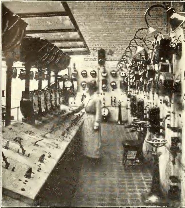
BRITISH PRACTICE—WOMAN SWITCHBOARD ATTENDANT
