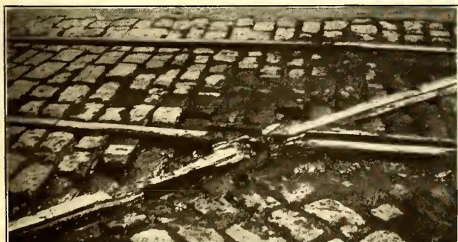
FIG. 3—FROG AND WING RAIL BADLY IN NEED OF REPAIR
