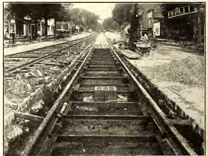
NEW TRACK BUILT ON OLD CONCRETE FOUNDATION, SHOWING TRACK HELD IN POSITION BY WOOD BLOCKS
