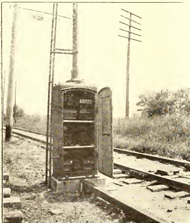
T. H., I. & E. SIGNALS—FRONT VIEW OF RELAY EQUIPMENT
