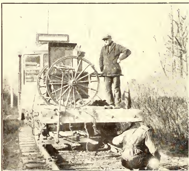
GENERAL VIEW OF ELECTRICAL BONDING OUTFIT
