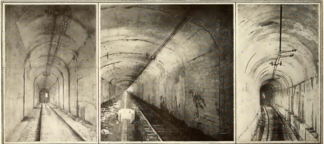
CANADIAN NORTHERN OVERHEAD CONSTRUCTION—OVERHEAD IN MONTREAL TUNNEL—LEFT, SECTION INSULATION AND ANCHORAGE AT PORTAL (TWIN-ARCH SECTION); MIDDLE, IN SINGLE-ARCH SECTION; RIGHT, ON CURVE IN TWIN-ARCH SECTION
