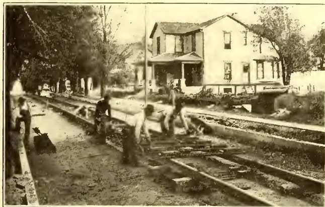
SEVEN MEN, PREPARING TRACK, KEEP AHEAD OF CONCRETE MIXER AND SIXTEEN MEN
