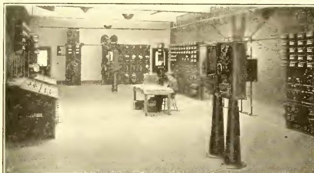
FIG. 6—SOUTH END OF WINDSOR PLANT OPERATING ROOM
