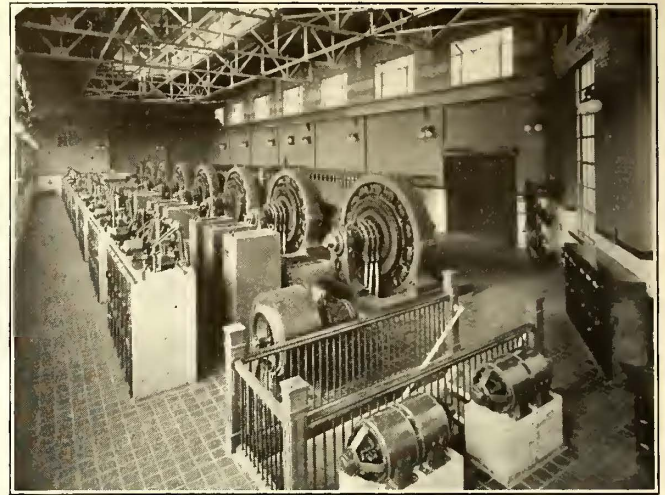
ALTERNATING-CURRENT ENDS OF THE ROTARY CONVERTERS AND ROWS OF CONTROL APPARATUS
