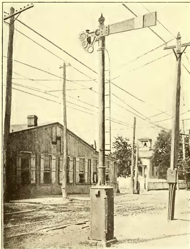
FIG. 14.—ELECTRICALLY OPERATED CROSSING DERAIL AND SEMAPHORE SIGNAL
