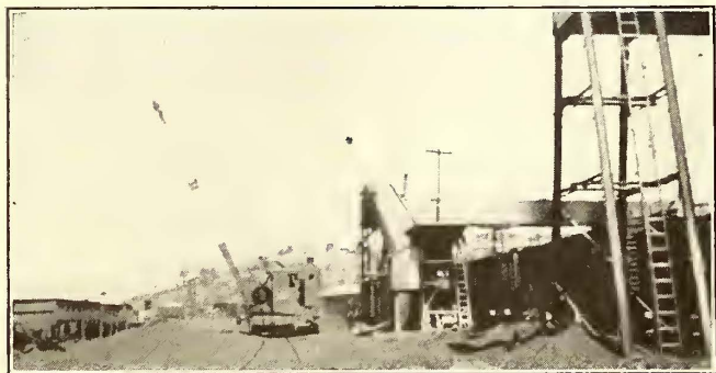
FIG. 1—CRANE AT WORK TRANSFERRING COAL FROM CARS TO CRUSHER.
