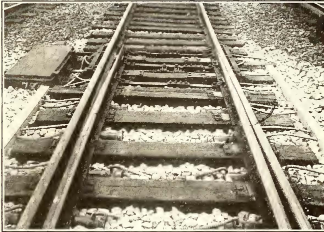
SWITCH WITH ELECTRIC SNOW MELTERS INSTALLED IN BALLAST
