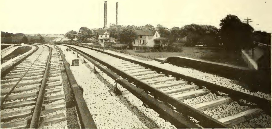
TIES MAINTAINED LIKE THIS HAVE A LONG LIFE
