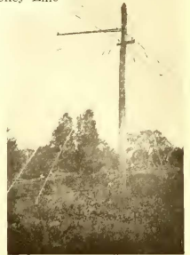
Four-Way Storm Guy on Trolley Line
