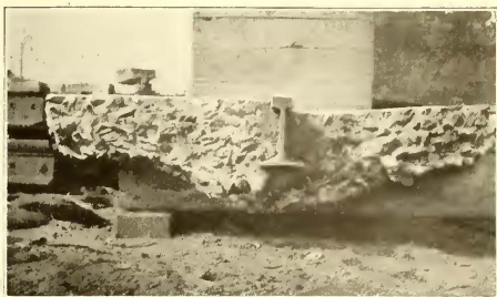
THIS SECTION SHOWS THE ADHESION OF THE CONCRETE TO THE RAIL
