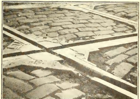
BROKEN RAIL HEAD IN CROSSING FROG
