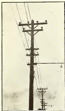
33,000-VOLT TRANSMISSION LINE WITH WOODEN BRACES FOR ARMS
