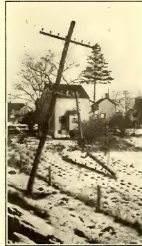
ARMS PULLED OFF POLE BY SLEET LOAD
