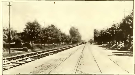
TEMPORARY DOUBLE TRACKS IN PLACE PREVIOUS TO REMOVAL OF MAIN TRACKS ON OCEAN AVENUE, BROOKLYN
