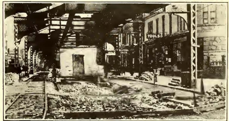
MAIN TRACKS REMOVED AND TEMPORARY SINGLE TRACK IN PLACE DURING CLASSON AVENUE SEWER CONSTRUCTION
