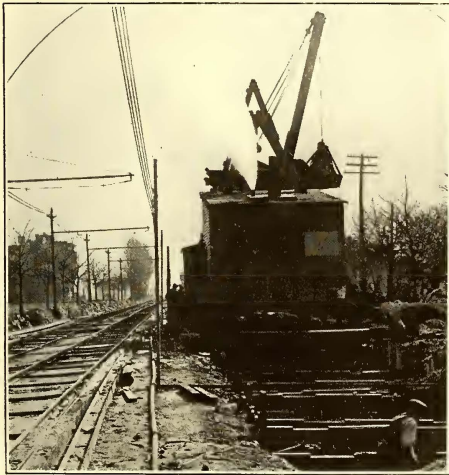
SEWER WORK IN PROGRESS, TEMPORARY TRACKS AND OVERHEAD WIRES INSTALLED AT SIDE
