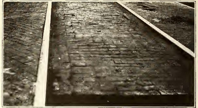
BUCKLED PAVEMENT ON STATE ST., BRIDGEPORT, CONN.
