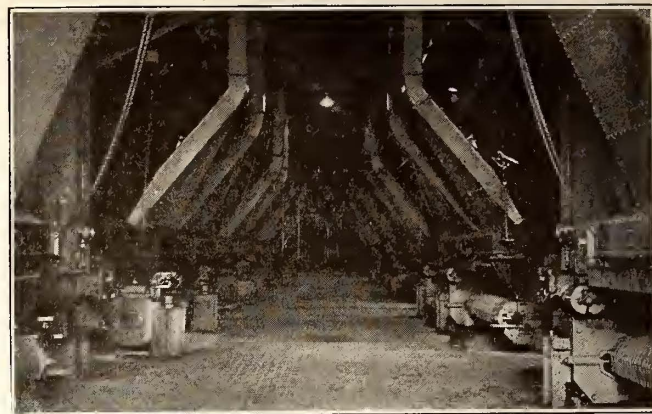
FIRING AISLE OF THE NEWPORT STATION BOILER ROOM
