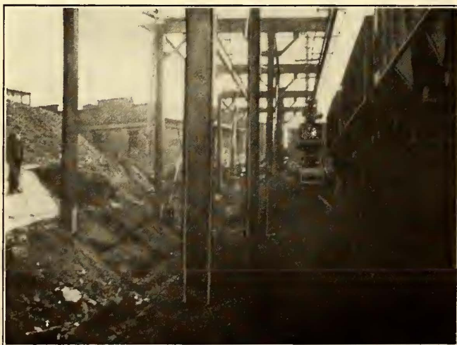
LOOKING TOWARD THE STREET FROM THE REAR END OF THE COAL STORAGE AREA
