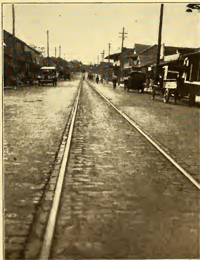
A STRETCH OF TRACK AND PAVEMENT ON NINTH AVE. STILL IN USE AFTER TWENTY YEARS
