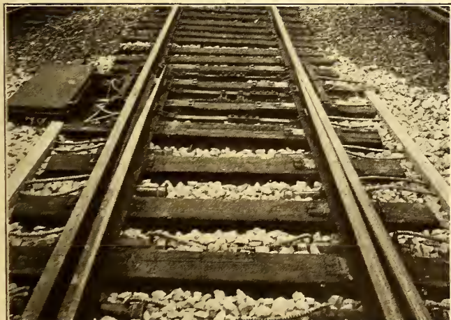
THE ELECTRIC SNOW MELTERS ARE INSTALLED AT SWITCH POINTS IN THE BALLAST UNDER THE RAIL
