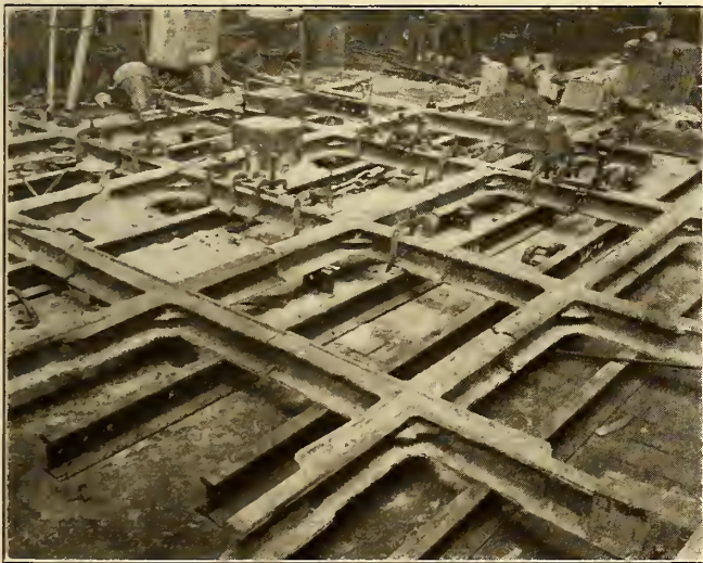
ASSEMBLING THE CHROME NICKEL STEEL CAST CROSSES, AFTER MACHINING, FOR WELDING THE JOINTS
