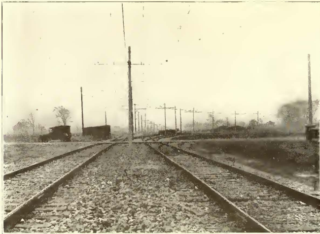
VIEW OF NEW LINE AT JUNCTION POINT WHERE SURFACE CONSTRUCTION BEGINS, SHOWING CENTER POLE AND CATENARY OVERHEAD CONSTRUCTION
