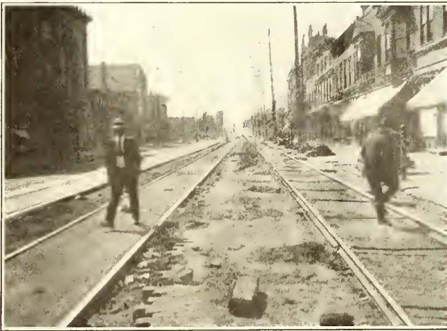
A STRETCH OF NEWLY LAID TRACK IN CLEVELAND THE TRACK AT THE RIGHT IS TEMPORARY
