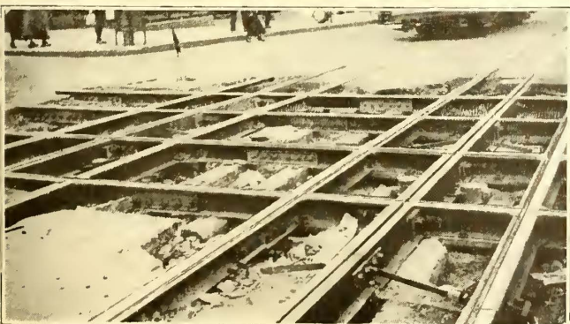
NEW CROSSING WITH THERMIT-WELDED RAIL JOINTS AND ARC-WELDED RAIL AND SLOT JOINTS
