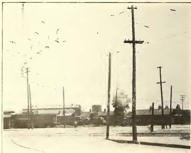
A 507-FT. TROLLEY GUARD INSTALLED ON A CONTINUOUS CURVE OVER THIRTEEN STEAM ROAD TRACKS
