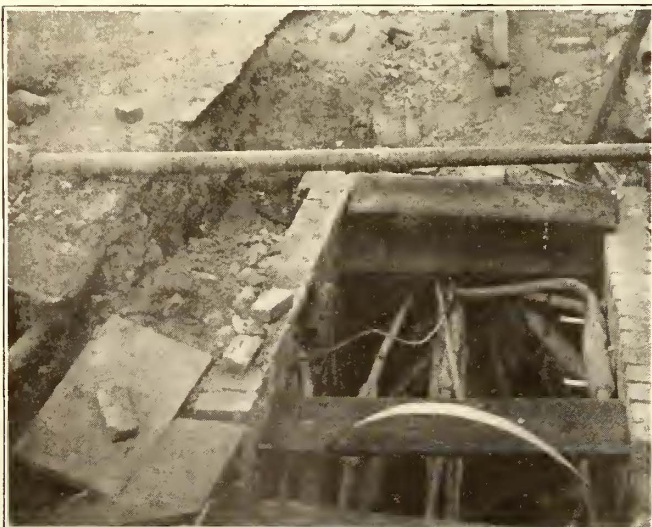
MANHOLE MOVED BY UTILITY AT A COST OF $2,000, AS RESULT OF STREET DEVELOPMENT FIFTEEN YEARS AFTER INSTALLATION. ILLUSTRATION OF "SUPERSEDECENCE"
