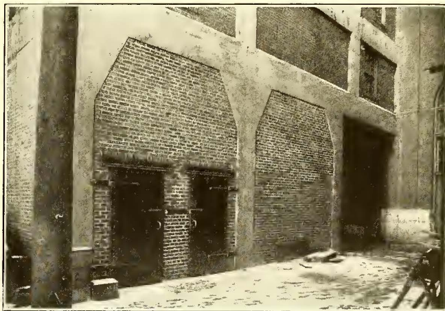
FIREPROOF STOREROOM AT WINSTANLEY POWER HOUSE PROVIDED BY BRICKING IN THE SPACE UNDERNEATH THE HIGH-TENSION SWITCHING ROOM
