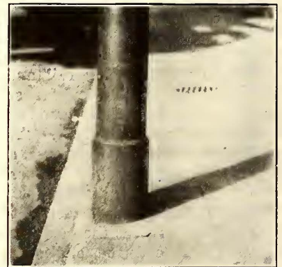
SLEEVE REINFORCEMENT OVER RUSTED PORTION OF STEEL POLE
