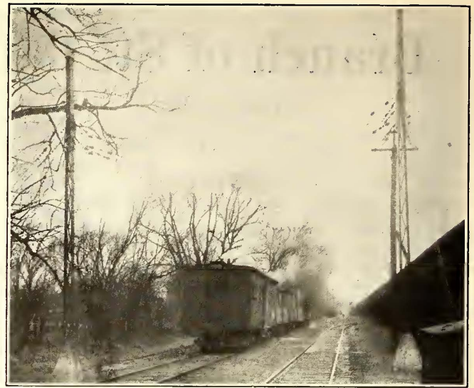
METHOD OF DEAD-ENDING HEAVY OVERHEAD—END POLES ARE GUYED TO 2-TON CONCRETE BLOCK ANCHORS BURIED IN THE GROUND
